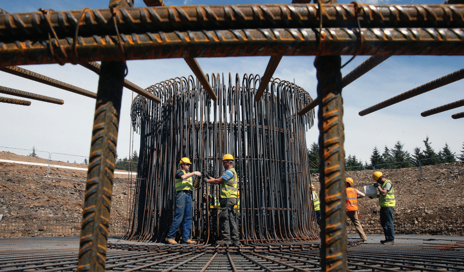
CELSA Steel UK is used to construct Pen Y Cymoedd Wind Farm (Source: CELSA Steel UK)
